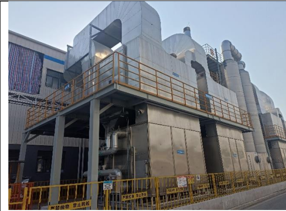
DA001 涂布废气排放口
